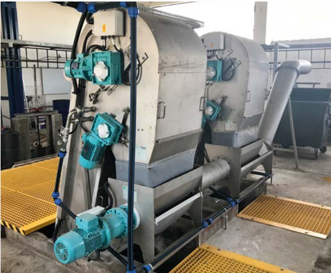
WWTP, Stupava, Czech Republic, 800_CP_1050 + LS_2400
