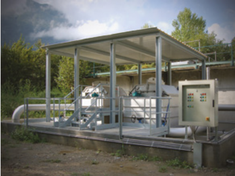
WWTP Carlazzo, Italy, 6FD_O
