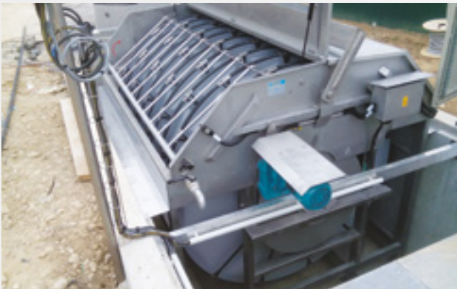
WWTP Ustaritz, France, 10FD_B
