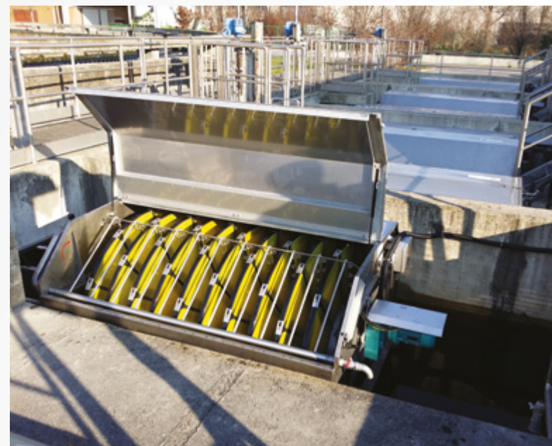
WWTP Ranica, Italy, 10FD_B
