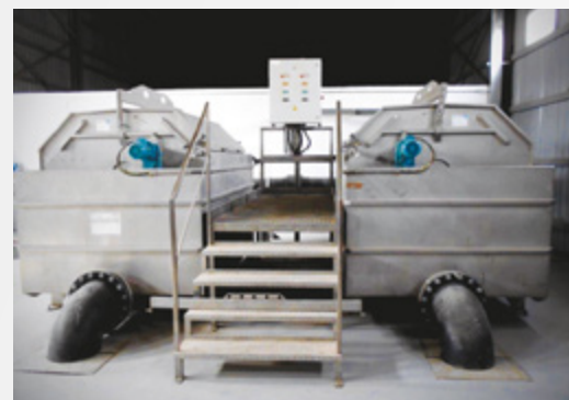
WWTP Al Kharj Industrial City, Saudi Arabia, 8FD_O_atyp
