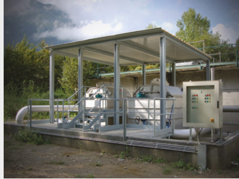
WWTP Carlazzo, Italy, 6FD_O
