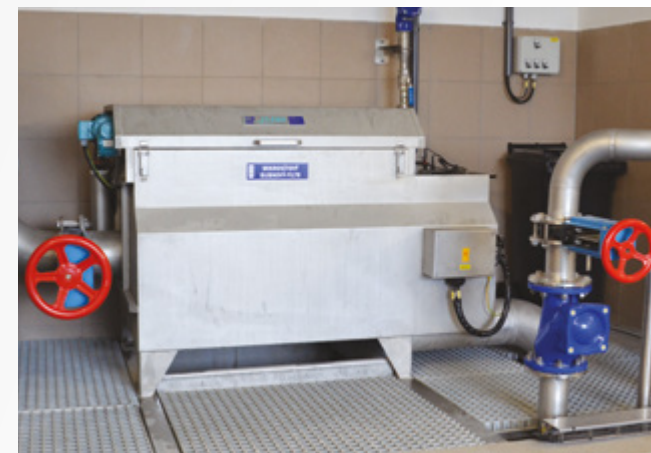
WWTP Chromeč, Czech Republic, 2FBO
