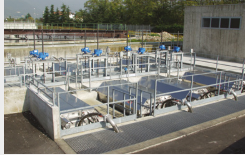
WWTP Ranica, Italy, 6FBB
